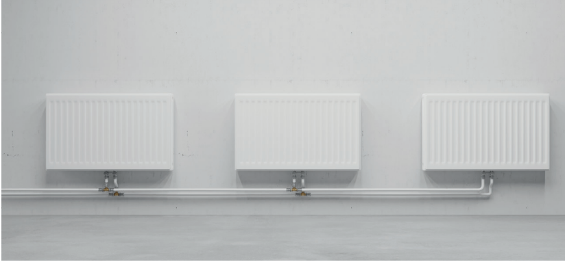
Fig. 46: Double pipe radiator heating.
