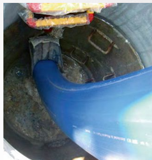
Japan, Osaka, DN250, Potable Water
