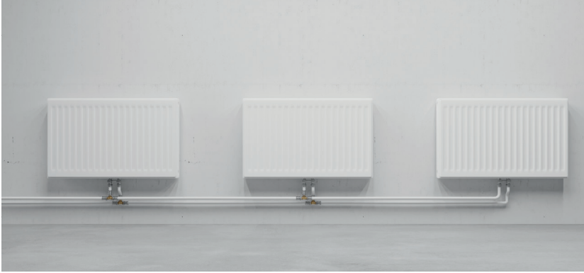
Fig. 46: Double pipe radiator heating.
