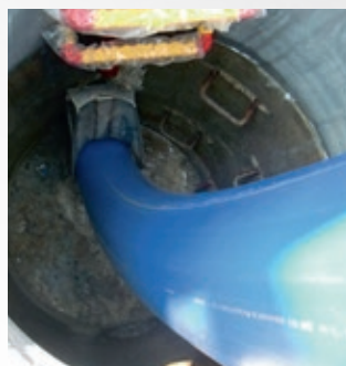
Japon, Osaka, DN250, eau potable
