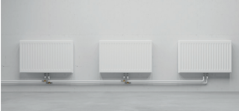
Fig. 47: Double pipe radiator heating.
